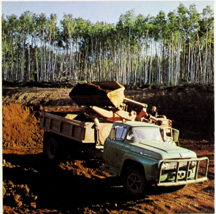
Strip mining ore near Hines Creek. This deposit promises to be the basis for a multi-million dollar steel industry in the Peace River area.
